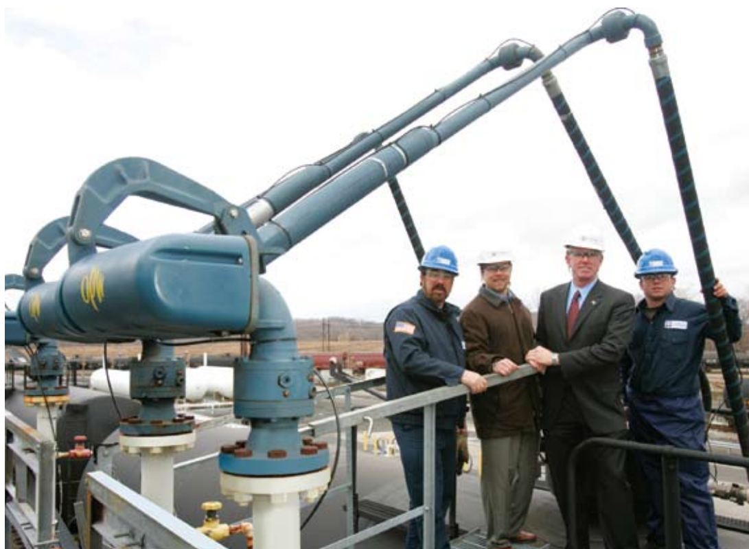
Larry Woodburn, Peter Gilman, Robert B. Nicholson III and Chris Bilancia stand on one of the LPG railcars at the Sparta Junction terminal. The OPW loading arms the company installed in 2006 have performed perfectly since day one.
