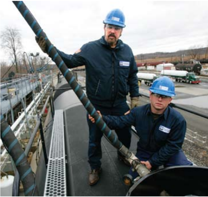
Larry Woodburn, Plant Manager, and Chris Bilancia, Operations Specialist, use the OPW loading arms every day to unload LPG from railcars from Targa Midstream Services, LP. They appreciate the ease-of-use and added safety the “A” frame loading arms provide.
